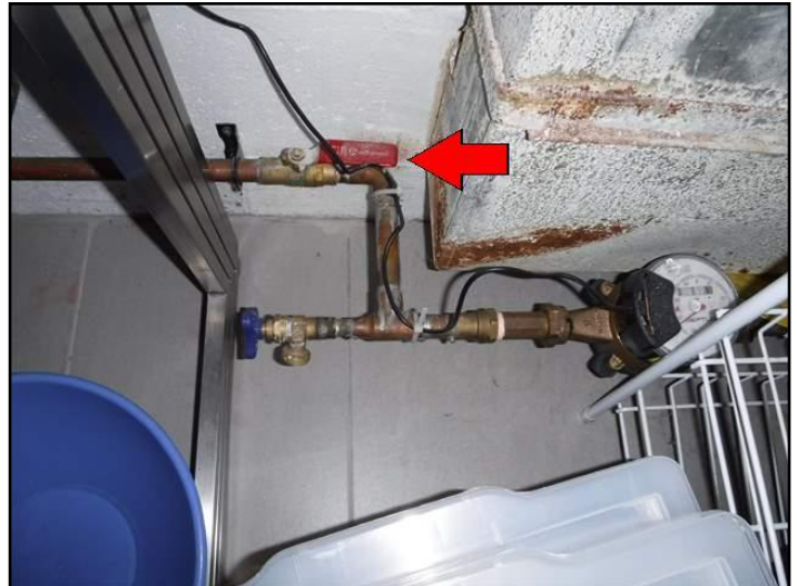
Secondary water shut-off valve
