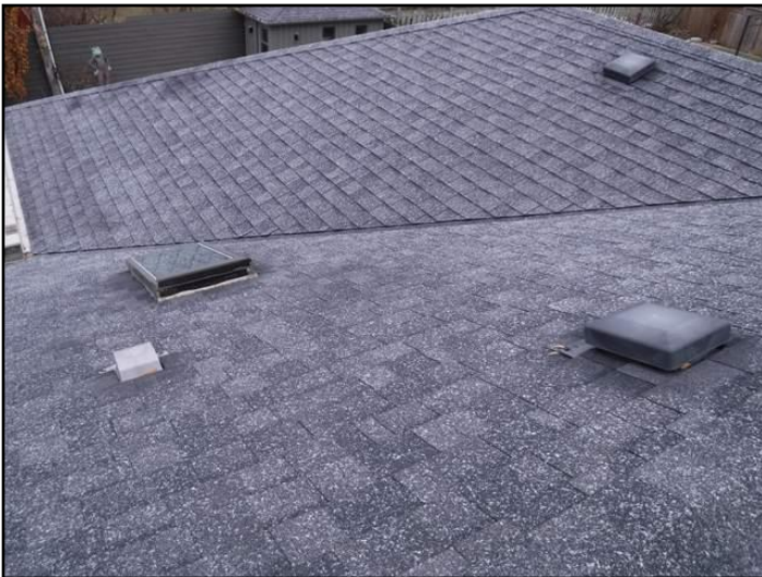
Asphalt shingle roof coverings wear out and...
