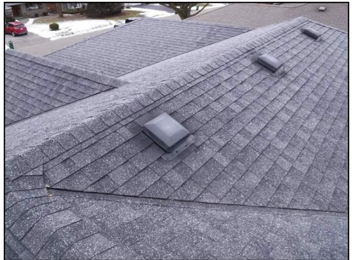
Asphalt shingle roof coverings wear out and...
