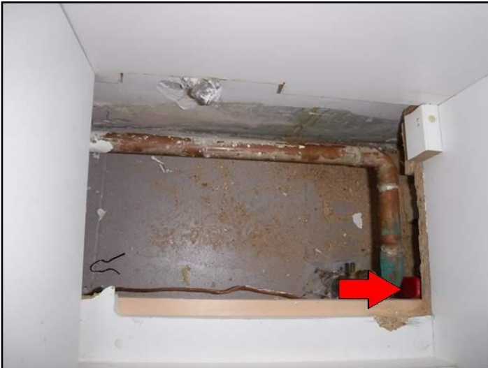
Main water shut-off valve
