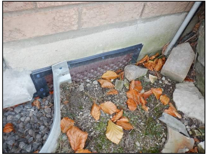
Drainage membrane/Prior repairs
