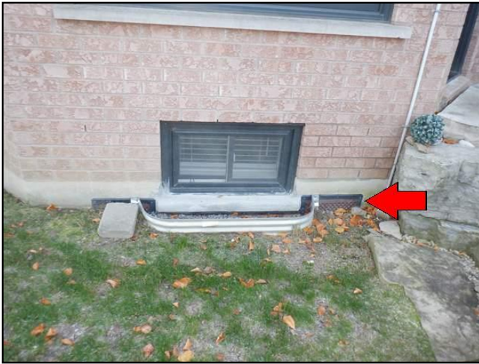
Drainage membrane/Prior repairs
