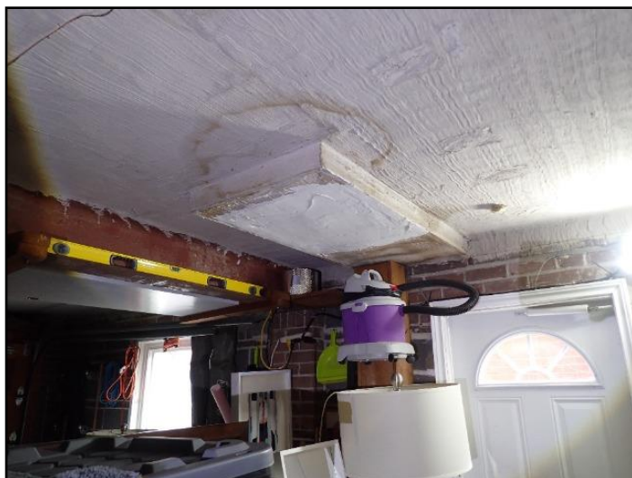
Stained/patched ceiling under Bathroom
