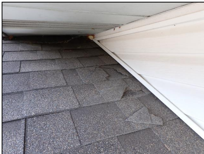
Damaged shingles under overhang
