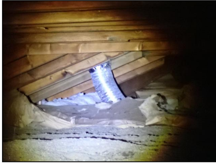
Ductwork not insulated in Attic
