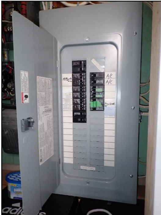
Panel and wiring are in good condition
