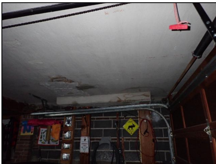
Stained/patched ceiling under Bathroom
