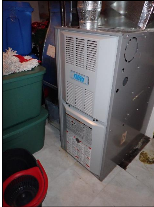
Furnace is approx. 20 years old
