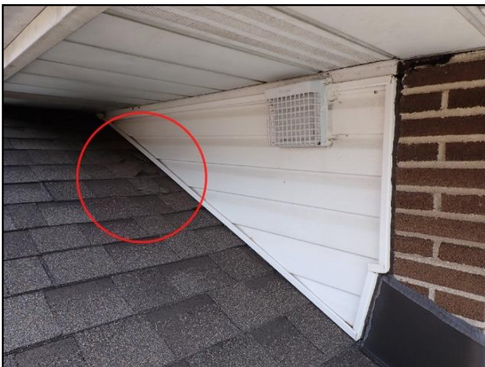
Damaged shingles under overhang
