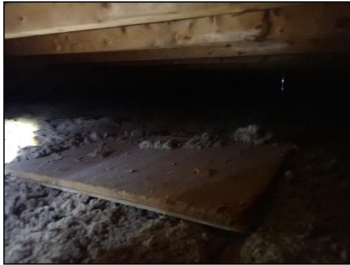
Access hatch not insulated
