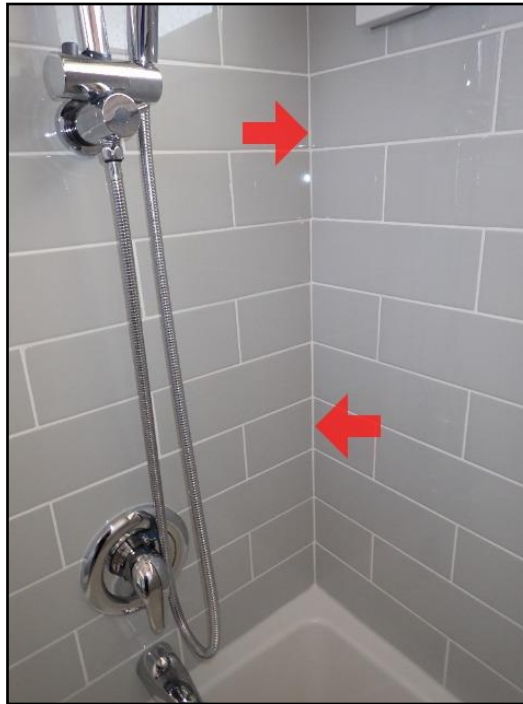
No caulking in corners
