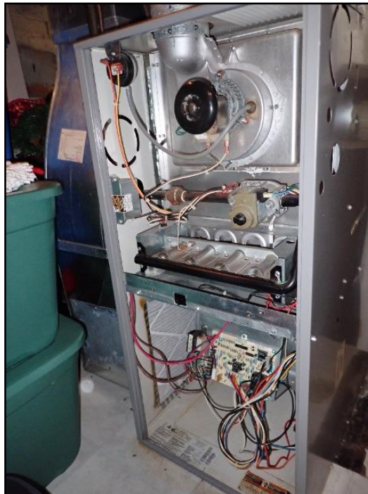
Furnace cabinet is in good condition
