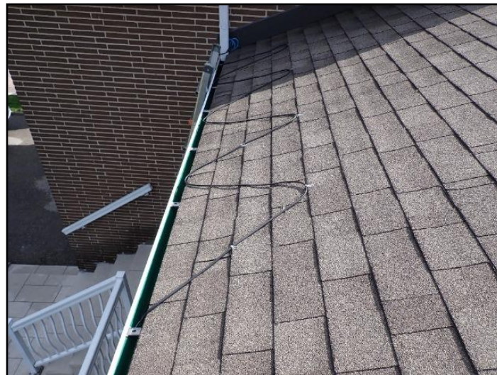
Ice melting cables over front entrance
