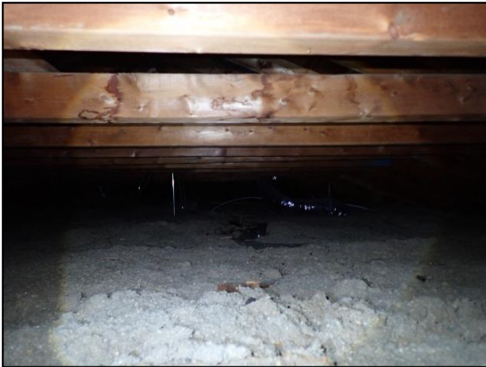
Attic insulation is below current standards
