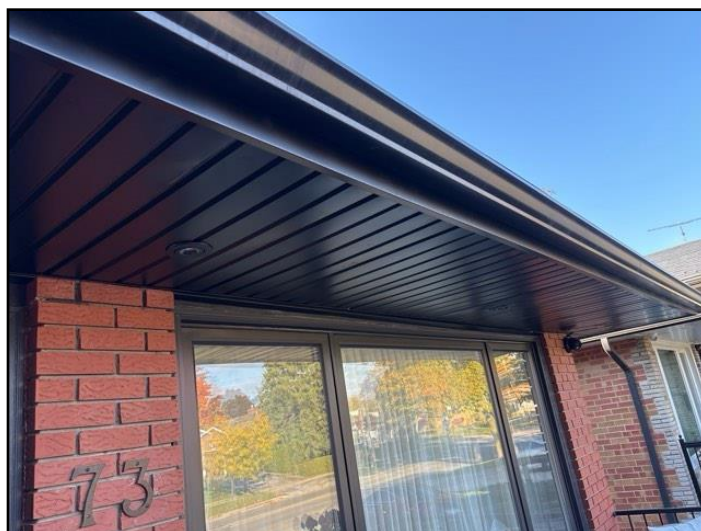
Vulnerable to ice damming
