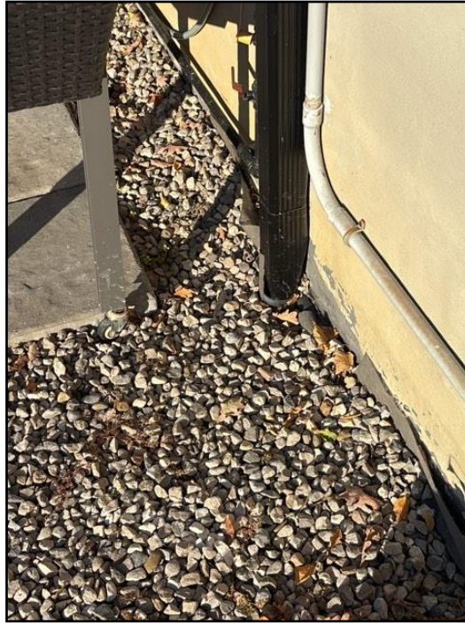
Discharge below grade
