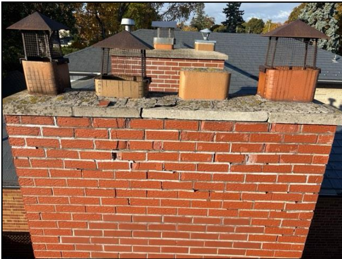
Loose, missing or deteriorated masonry
