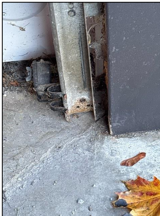
Sensors poorly located
