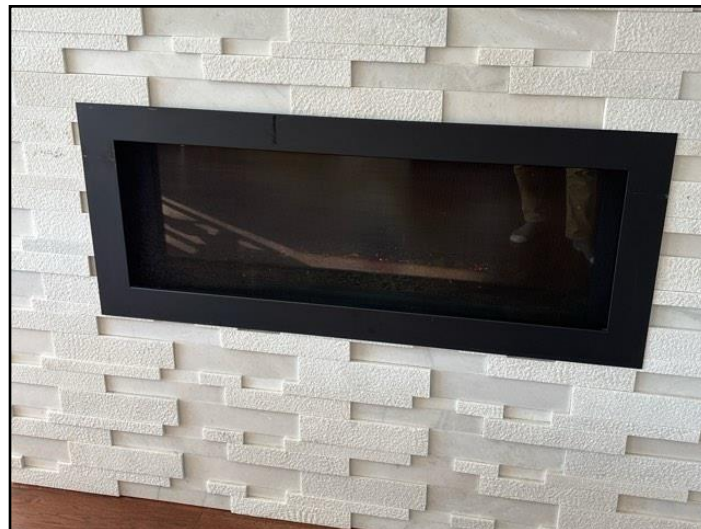
Gas fireplace check pre-use -
