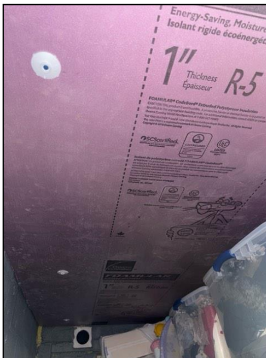
Combustible insulation exposed
