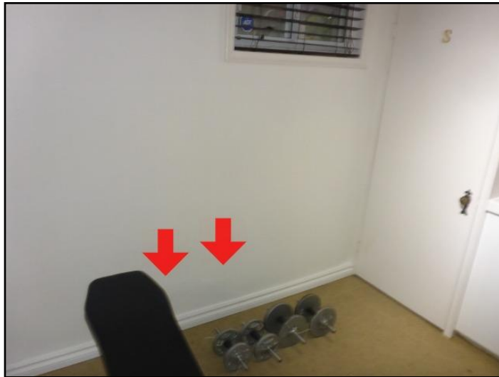
Patched area under window
