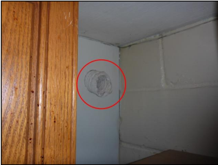
Discharges into furnace room
