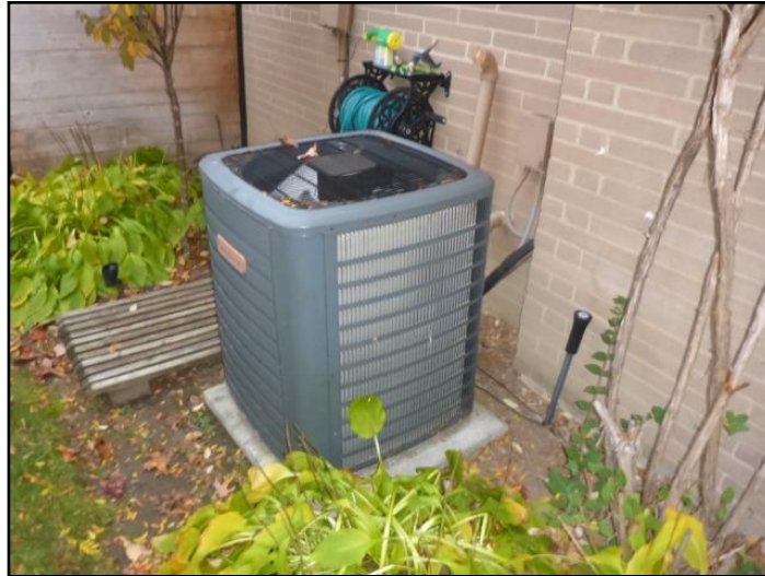
Air cooled- outdoor unit
