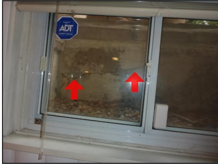
window well cracked
