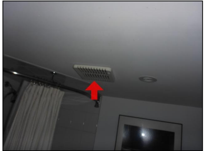
Does not discharge to exterior
