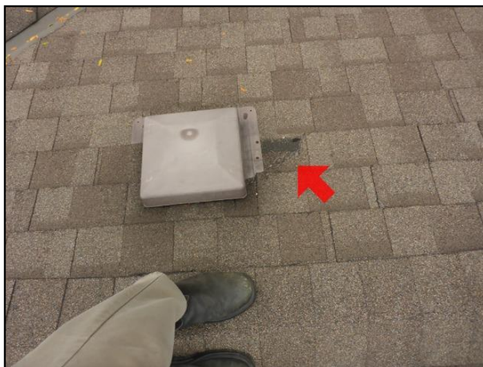
Damage- torn shingle
