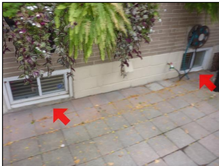
Missing window wells
