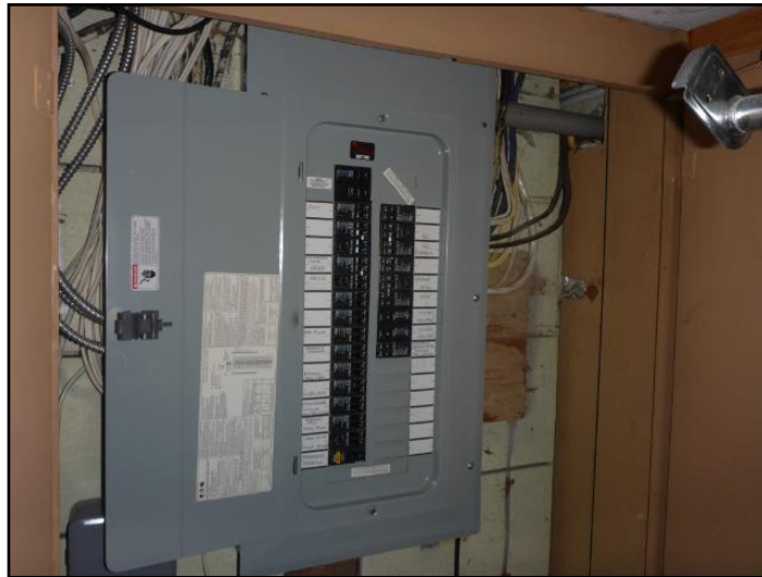
Some circuits not labeled
