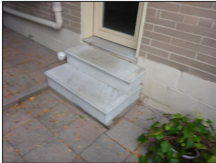
Trip hazard at uneven steps
