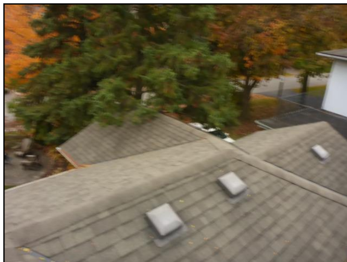
Tree branches touching roof
