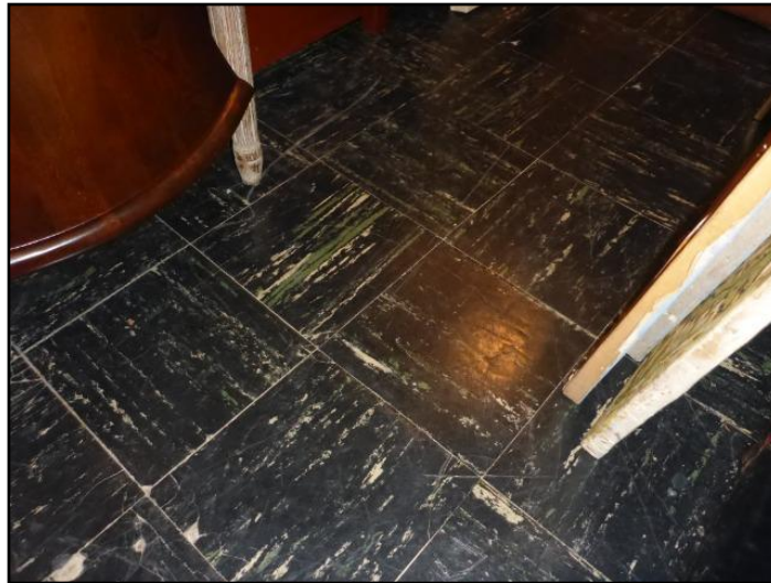
Old 9"x 9" resilient floor tiles noted
