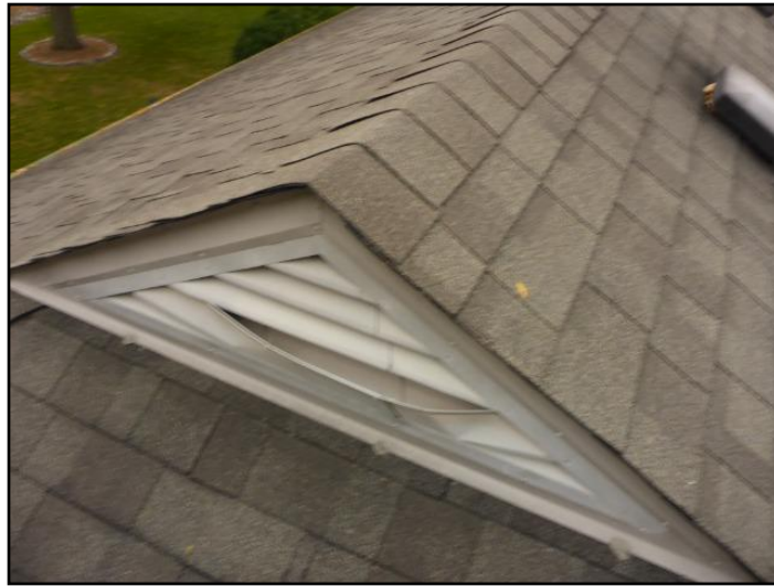
Animal activity noted (damaged louvers)
