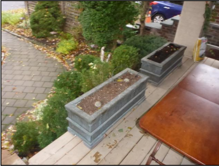
Missing railing at porch
