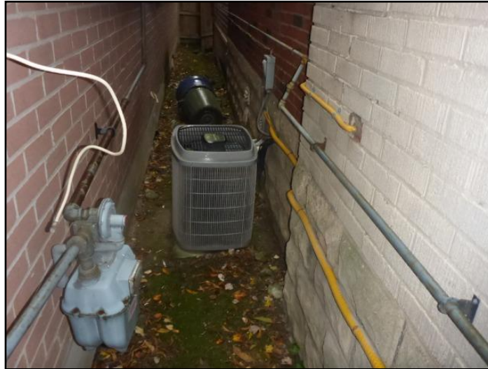
Air cooled- outdoor unit
