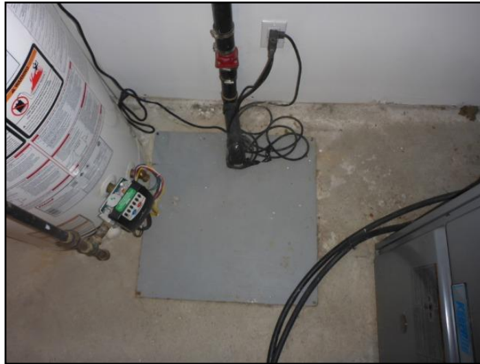
Sump cover not removed
