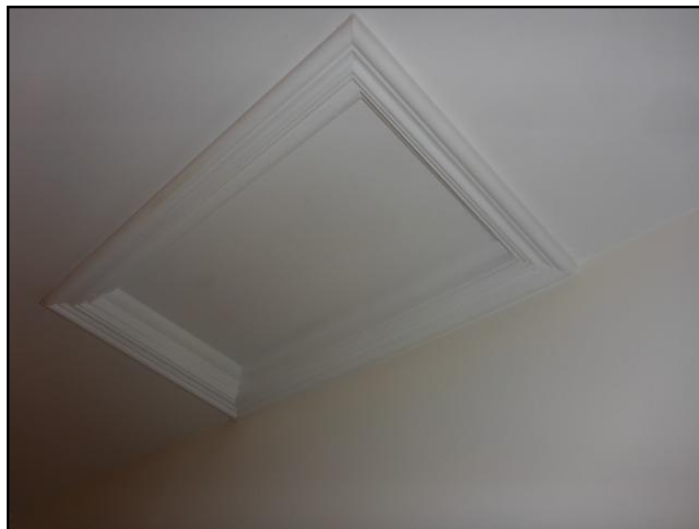
Access hatch painted shut
