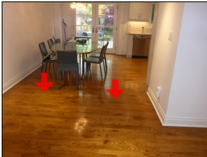
Hump in finished floor
