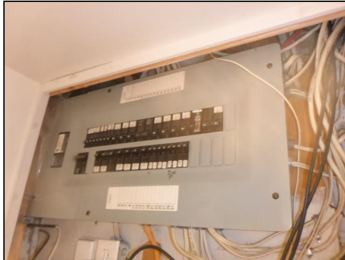
Circuits not labeled
