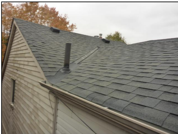
Vulnerable area- plumbing stack in valley
