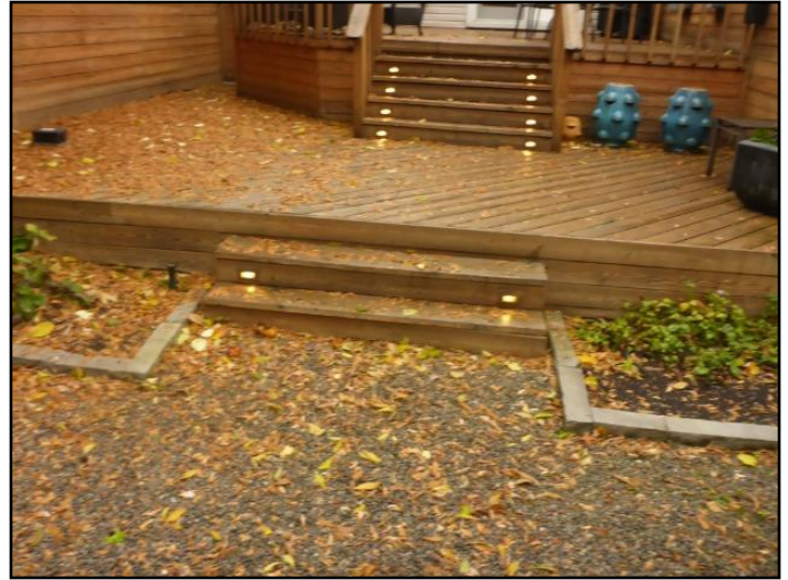
Missing railings at lower deck
