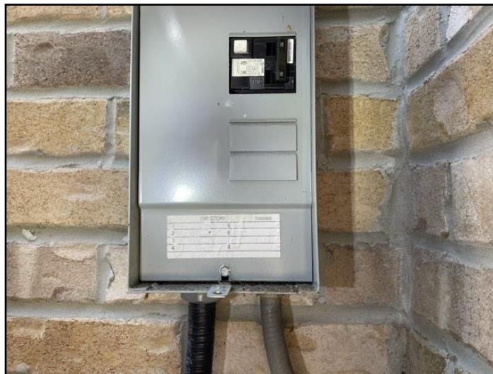
Breakers - hot tub
