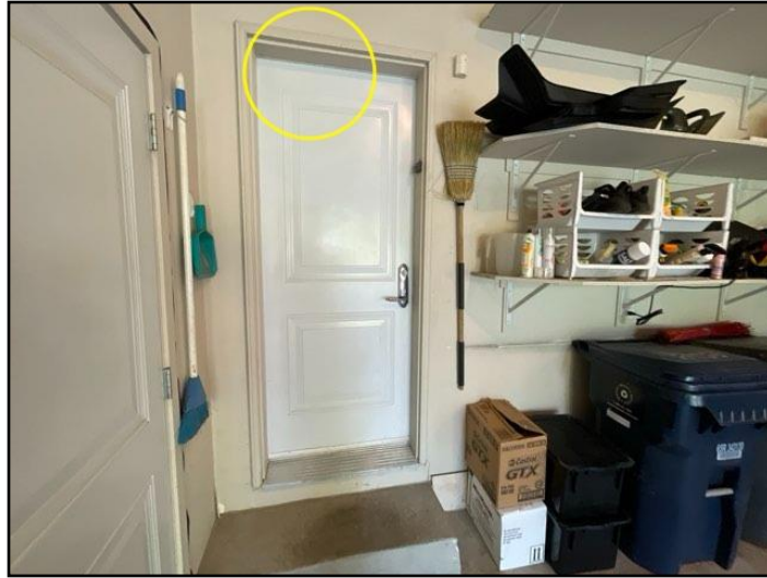
Door closer - missing
