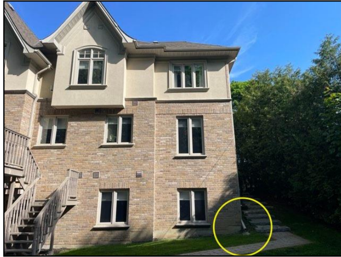
Discharge too close to building
