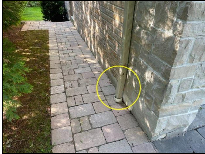
Toronto - Discharge below grade
