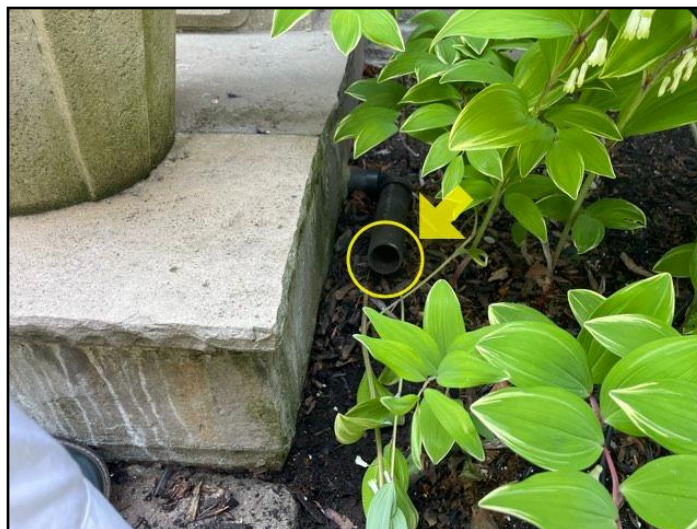
Discharges less than 6 feet from home
