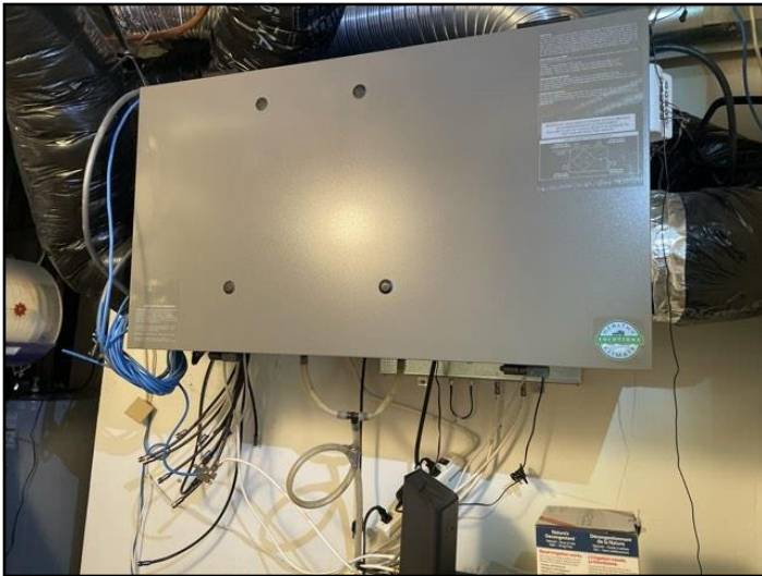
Heat Recovery Ventilator (HRV)
